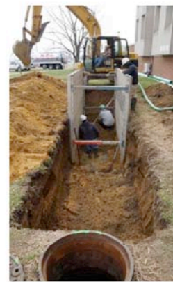
Safety box placed in trench to prevent sidewall caving while men prepare for sewer line replacement.
