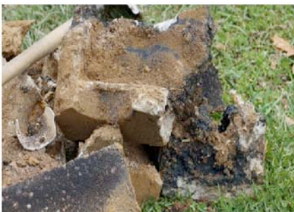
Crushed distribution box removed for replacement.
