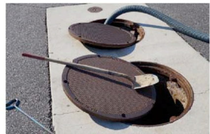
Grease trap lid removal for regular maintenance.
